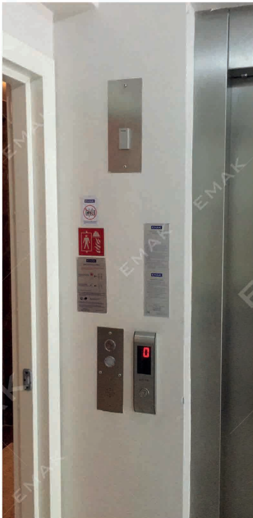
Keçiören / ANKARA 3 Elevators, 30 Stops, Rated Load: 1000 kg
