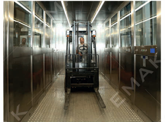
Çevik Warehouse - Showroom / ANKARA EMAK Hydraulic Cargo Elevator Rated Load: 4 Tons
