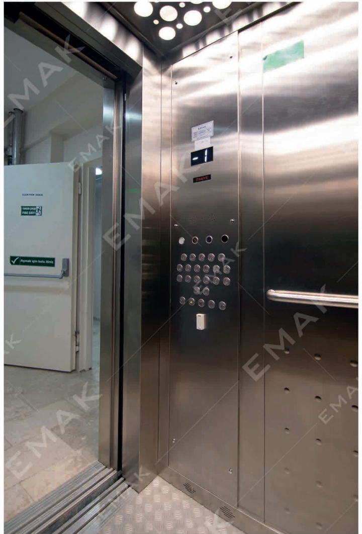
Agro Construction / İSTANBUL 7 Elevators, 19 Stops, Rated Load: 1200 kg
